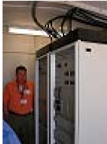
Processing units and VHF Transmitters Installed at Seatac
